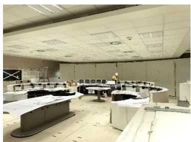
Main Control Rooms
